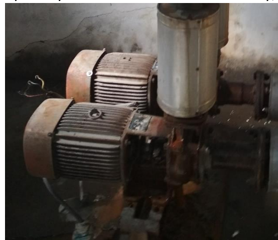
Figure 5: Old Chilled Water Pumps
